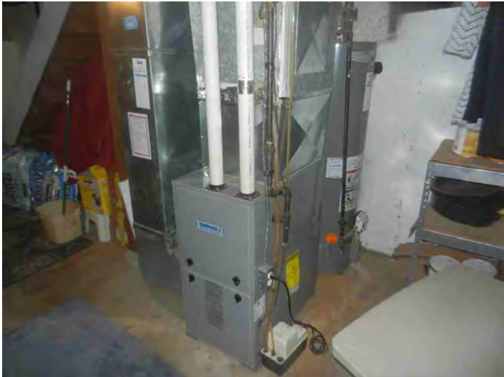
Furnace & water heater
