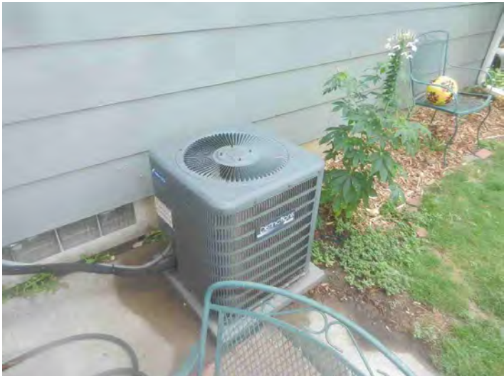
Central air unit
